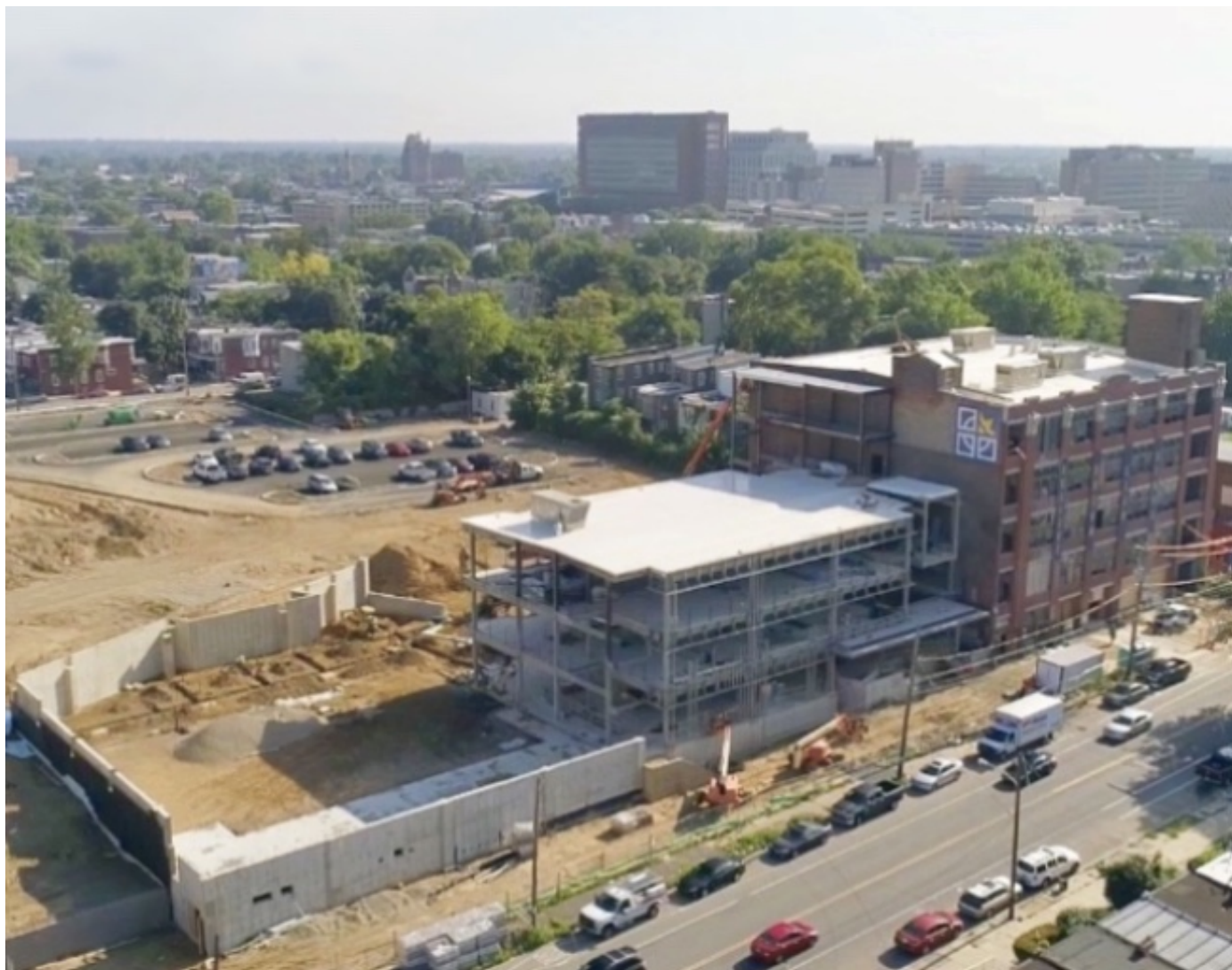
New school construction site makes continued progress, including the parking lot and foundations for the gym.
